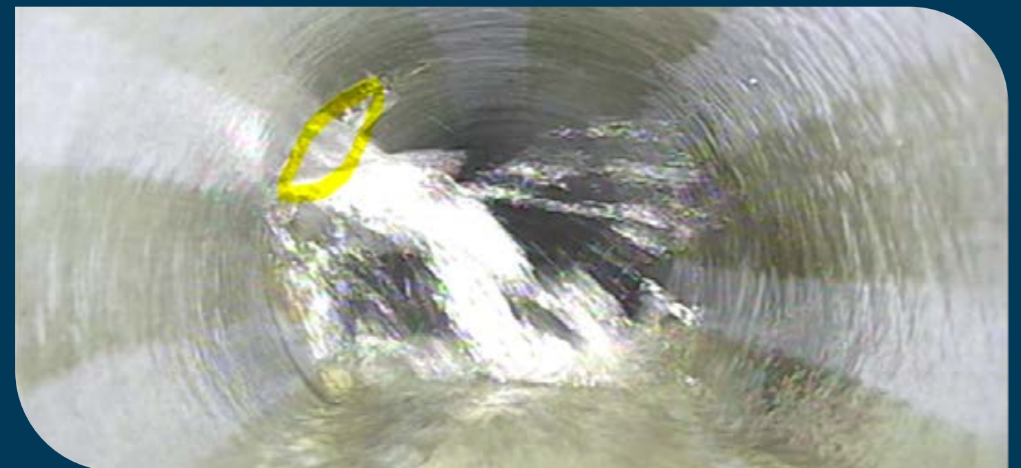
A source of inflow and infiltration from the wastewater lateral
