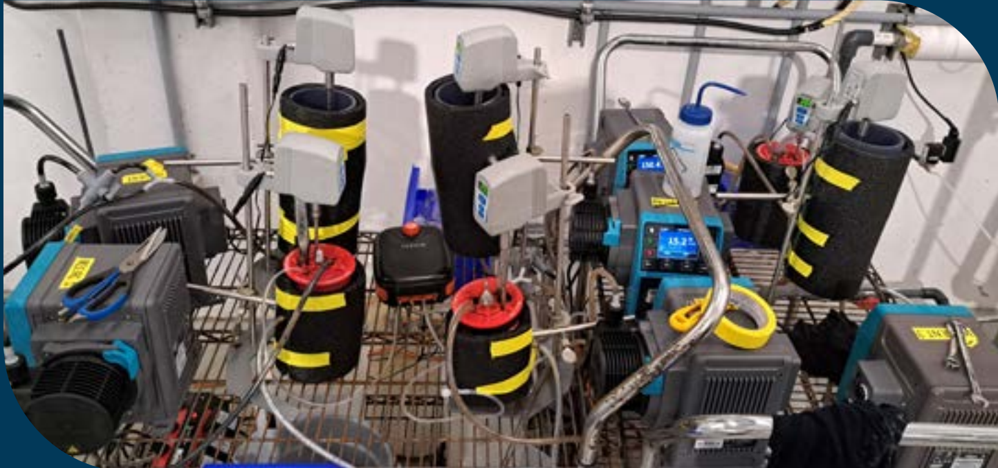
Biological Aerated Filtration (BAF) Pilot Testing
