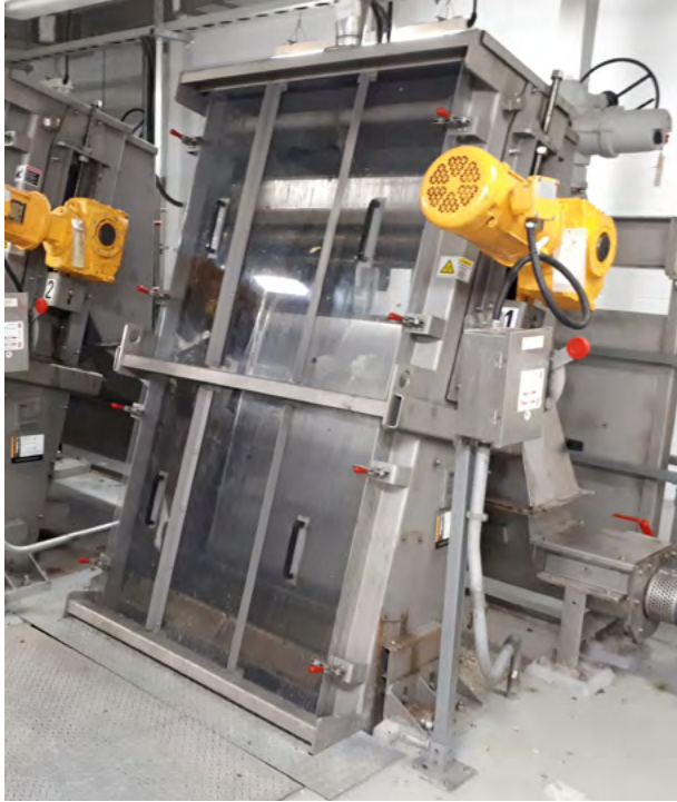
Herring Cove WWTF Fine Screens
