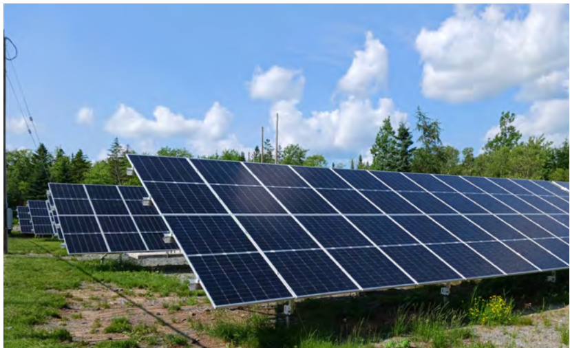
Aerotech WWTF Solar PV Panels
