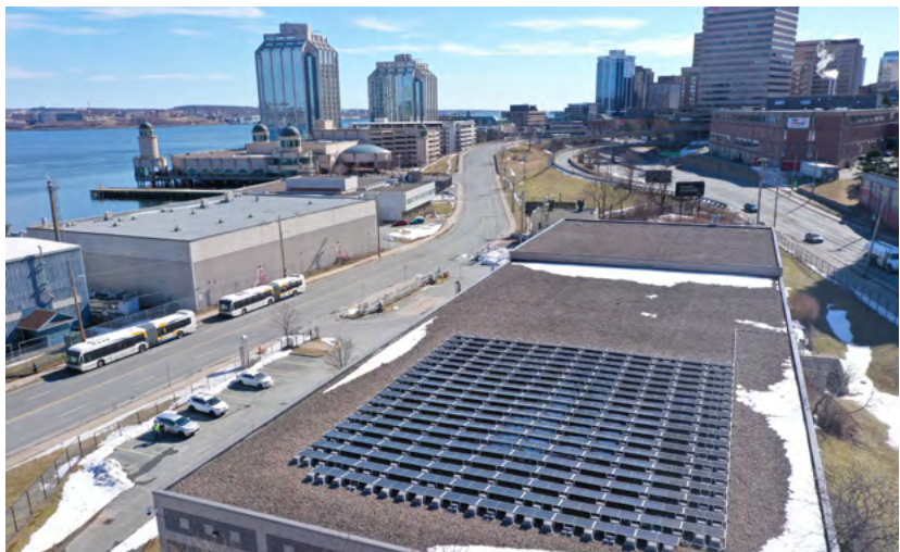
Halifax WWTF Solar PV Panels
