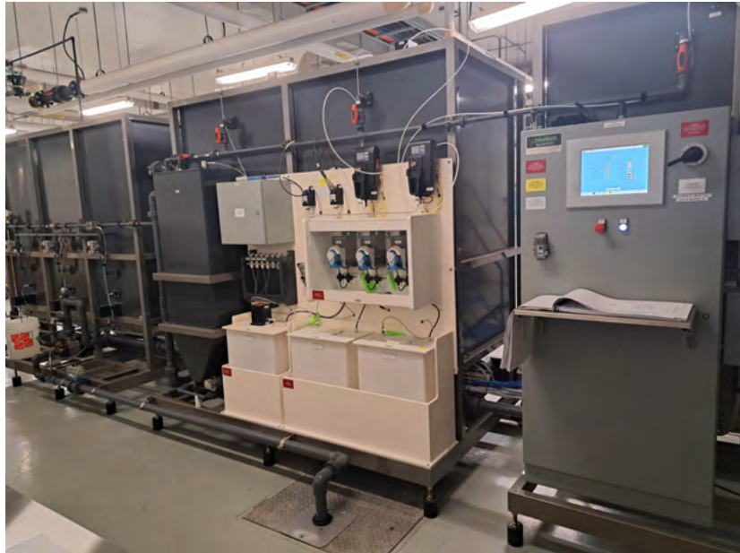
Large-Scale Pilot Plant
