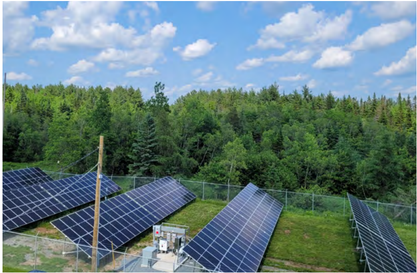
Aerotech WWTF Solar PV Panels
