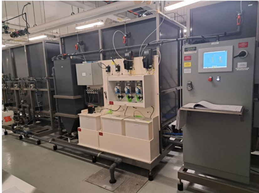
Large-Scale Pilot Plant
