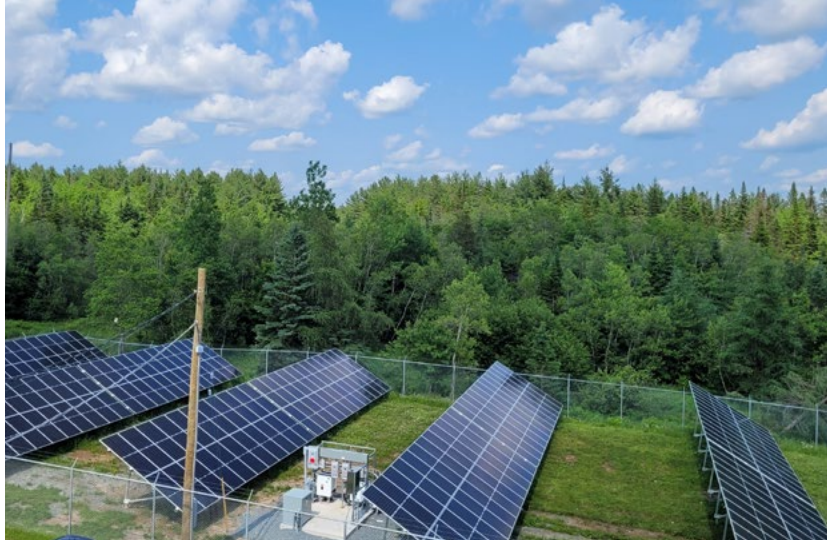
Aerotech WWTF Solar PV Panels
