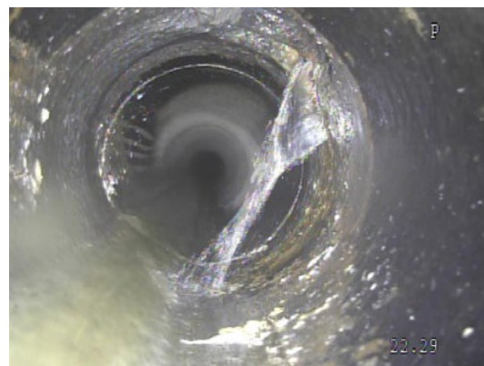
CCTV Image of Stormwater Entering the Wastewater System
