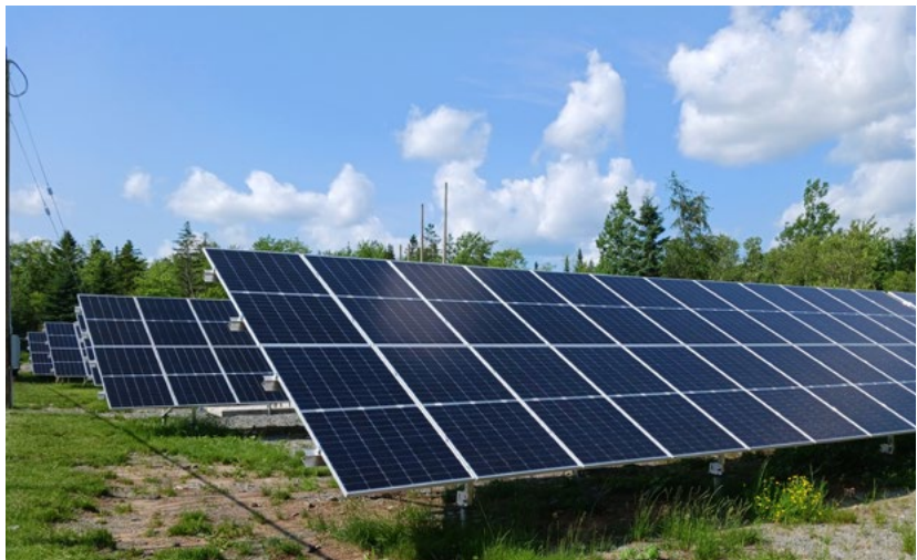
Aerotech WWTF Solar PV Panels
