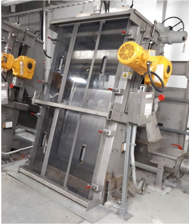
Herring Cove WWTF Fine Screens
