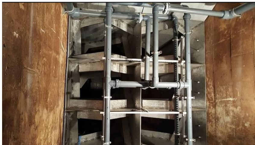
Figure 3.1: In-Channel Static Mixer
