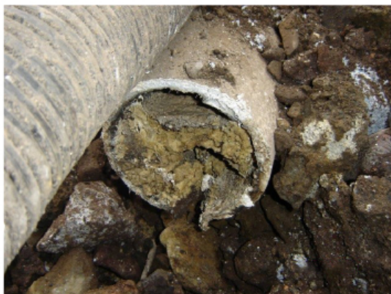
Solidified Fat, Oil, and Grease blocking a wastewater pipe.
