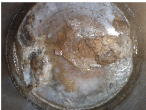
Manhole filled with grease and food debris.
