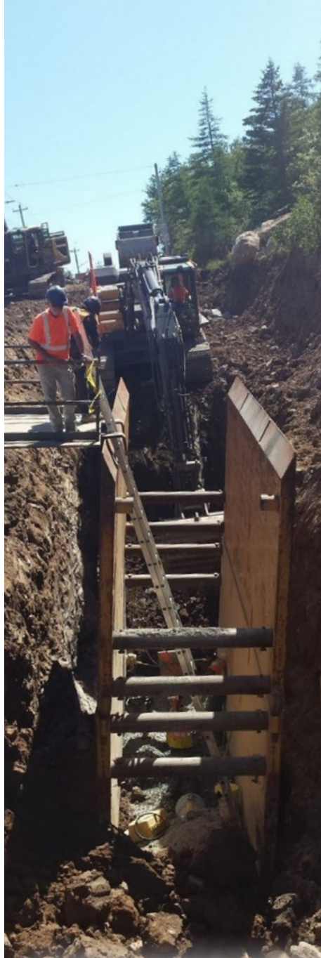
Leiblin Pump Station Elimination
