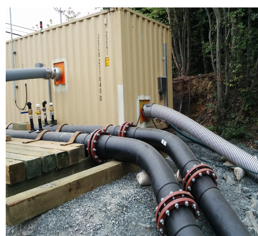
EXISTING SYSTEM ENCLOSURE AND SIPHON
