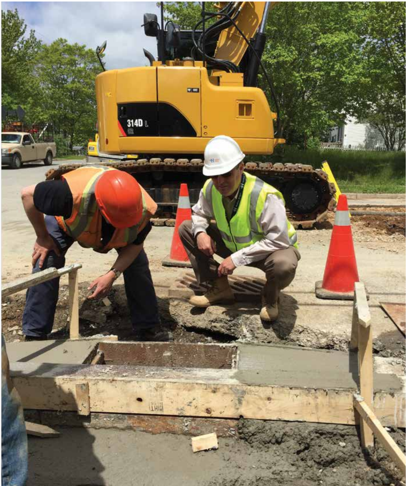
General Manager Carl Yates taking the safety message to the job site
