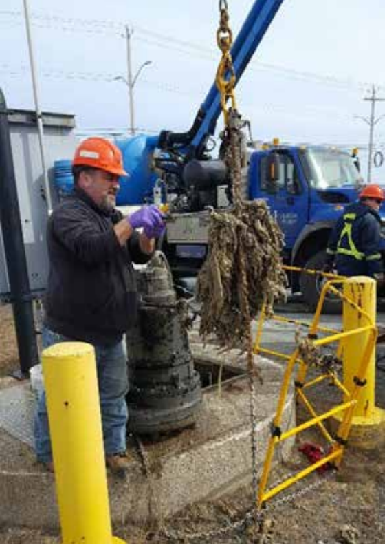
Wipes, FOG and other debris clogging the Susie Lake pumping station
