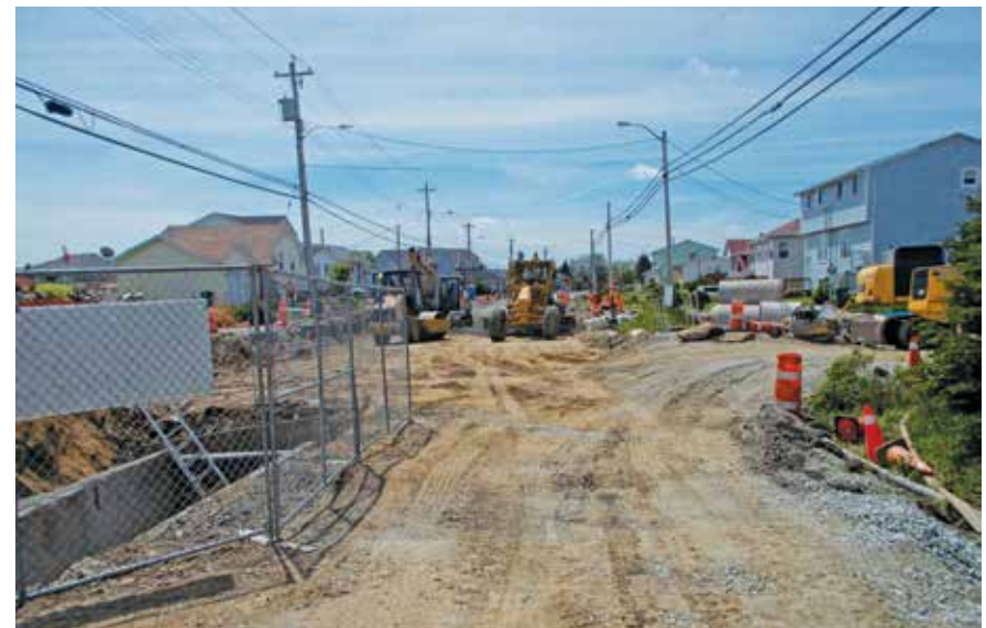
Cow Bay Road deep storm sewer project—getting stormwater out of the wastewater system
