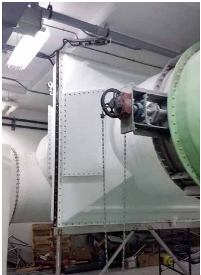
Heat recovery ventilation system at the Halifax WWTF
