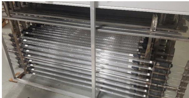
UV Light Bank removed from tanks for cleaning.
