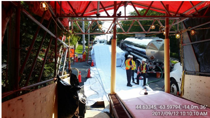
Pipe lining laid out in preparation for insertion in existing sewer pipe.
