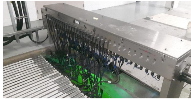
UV Light Bank actively disinfecting treated wastewater.
