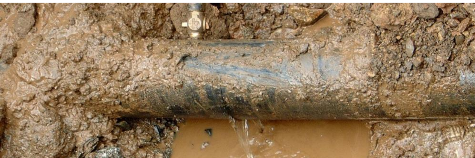
Water main leak detected and uncovered for a repair.
