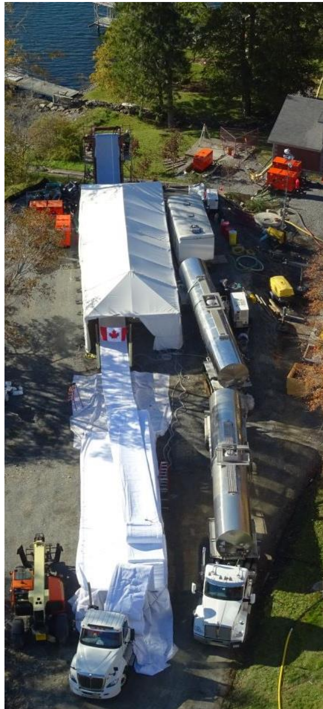
Aerial photo of the main point of access to the Northwest Arm Sewer Line.
