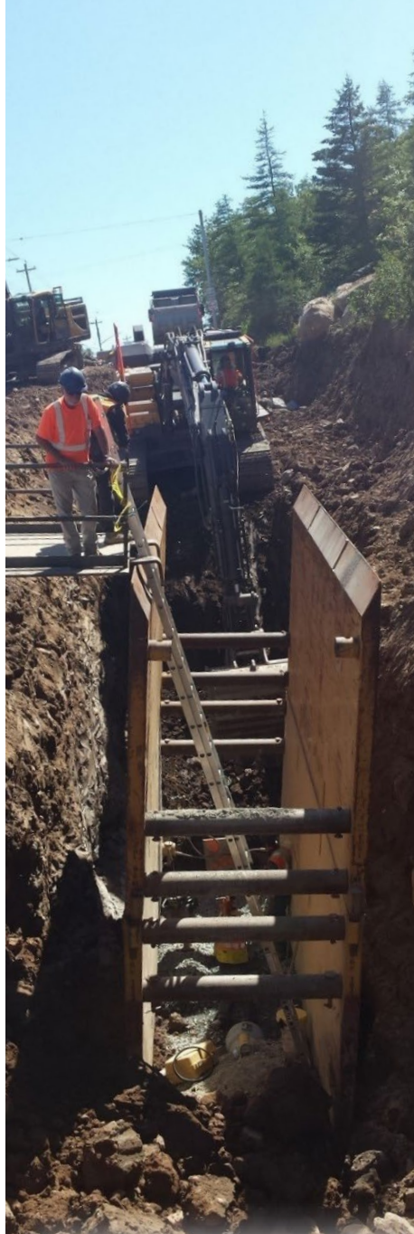
Leiblin Pump Station Elimination
